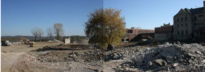
The late stages of demolition on site of the new Jefferson City Courthouse
